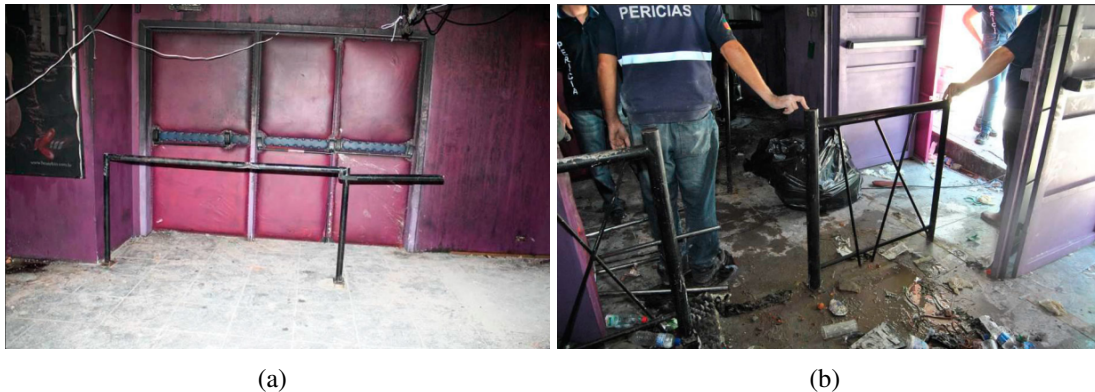
Figure 3 Images of some of the bars added by owners in the evacuation route near to exit of Boate Kiss. Additionally, in (a) the middle door was locked (images source: IGP-RS [16]).
