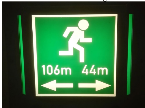
Fig 4. Evacuation signs with the distance to evacuation exits from the main tunnel
